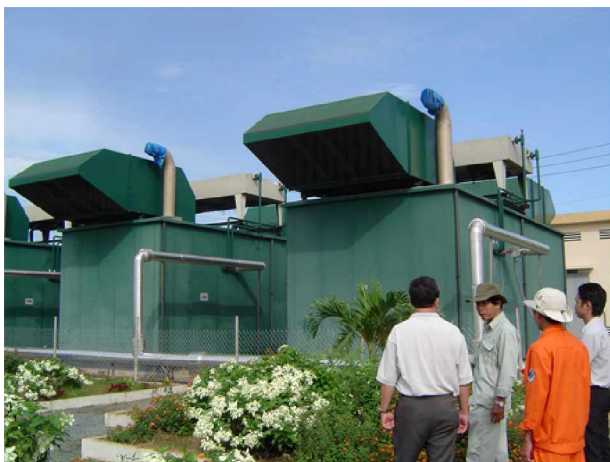
Power generation from landfill gas
