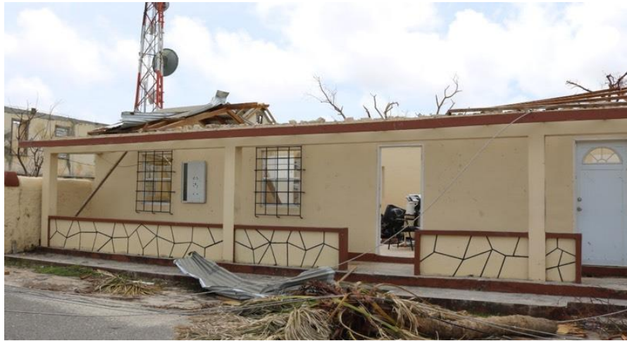
Figure 3: Office buildings in Barbuda left with no roof, destroying equipment and IT systems after the passage of Category 5+ Hurricane Irma in September 2017
