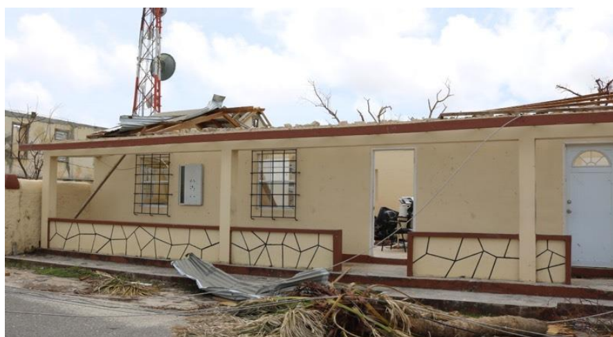
FIGURE 2. Office buildings in Barbuda left with no roof, destroying equipment and IT systems after the passage of Category 5+ Hurricane Irma in September 2017
